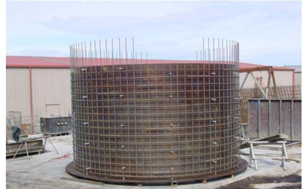
4m Diameter tank under construction. Due to the height required, the tank was slipped formed in 2 hours and weighs 23 tonnes
