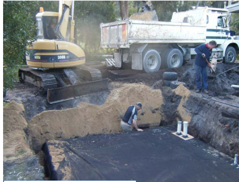
Retention Tank, Ansons Bay, NE Tas
