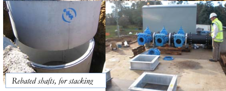
Beauty Point PS – Chris Temby, ready for in-situ pour of roof slab
