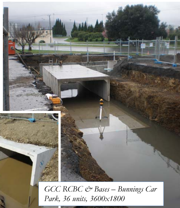
Osmaston Dual RCBC & Bases - MVC
